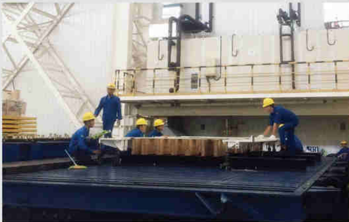
Assembly Workshop facility galleries
