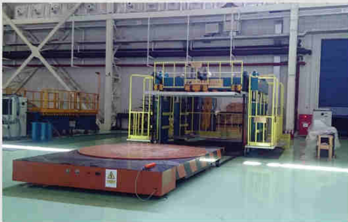
Winding Workshop facility galleries
