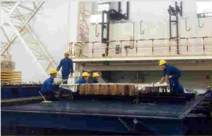
Assembly Workshop facility galleries
